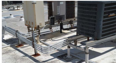
Corrosion on Anchors
